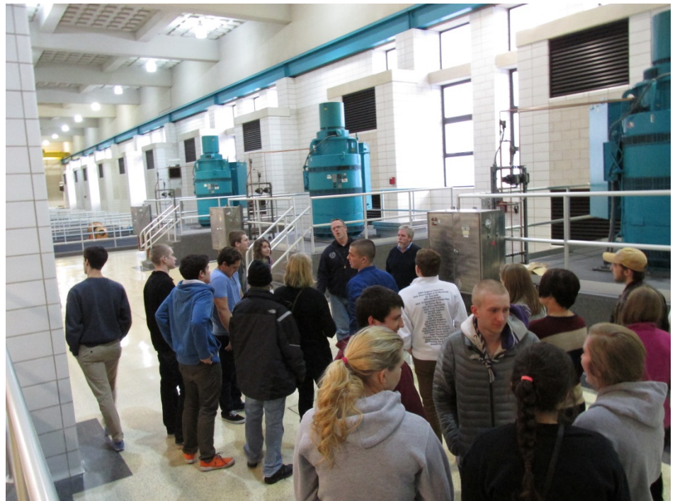
Mike Weed explaining why the motors are elevated separately from the pumps
