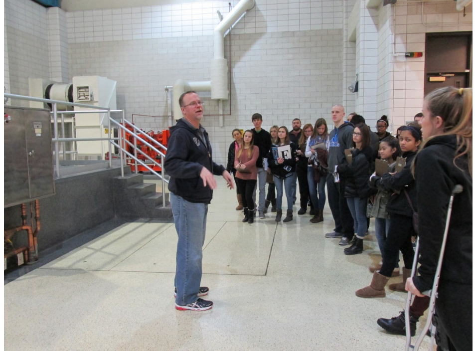
Weed explaining why the motors are elevated separately from the pumps
