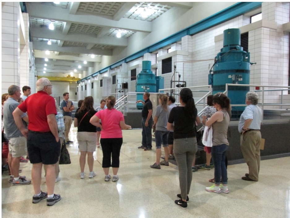
Weed explaining how the motors turn the pump impellers to move water through the pipes
