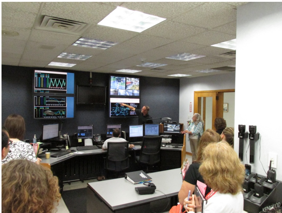
Mike Weed presenting DWC's SCADA system in the control room
