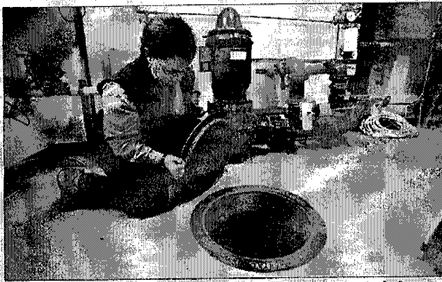
Jill Stites opens the Ryerson Woods Nature Preserve cistern that holds rainwater for fire suppression and, with state permission, toilet flushing. CHRIS WALKER/TRIBUNE PHOTO
