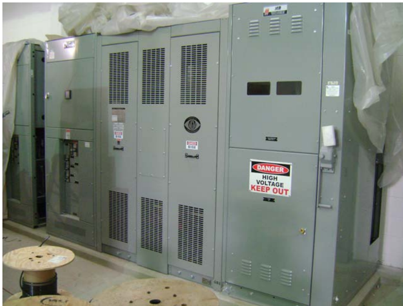
Power Distribution Panels in Electrical Room
