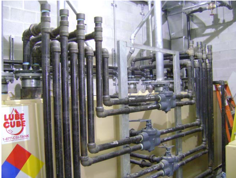
Fuel Piping in Day Tank Room
